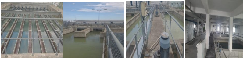
Fig. 5. Barați Water Treatment Plant: Coagulation-flocculation stages, Lamella clarifier, Rapid sand filters and water– current state
