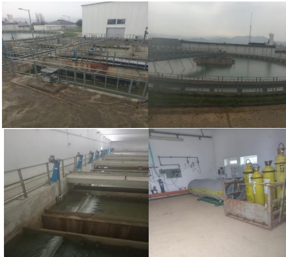
Fig. 3. Cărbăoaia Water Treatment Plant: Coagulation-flocculation stages, Radial clarifier, Rapid sand filters and water disinfection equipment.– current state
